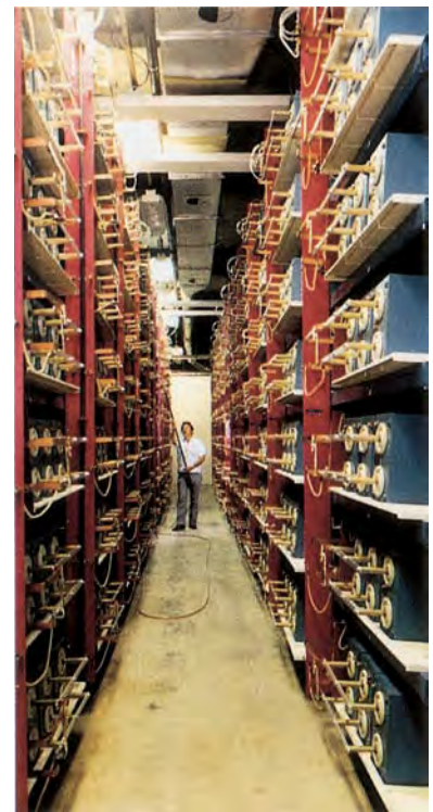
A capacitor bank for storing energy to be used by the pulsed Nova laser at Lawrence Livermore Laboratories. The laser is used in fusion studies. (Lawrence Livermore National Laboratory.)
