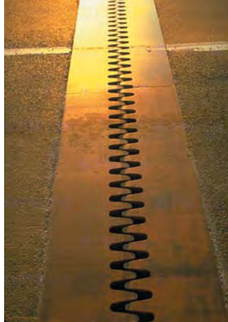
FIGURE 20-4 Expansion joints, such as this one, allow bridges to expand with increases in temperature. (Frank Siteman/Stock Boston, Inc./PictureQuest.)
